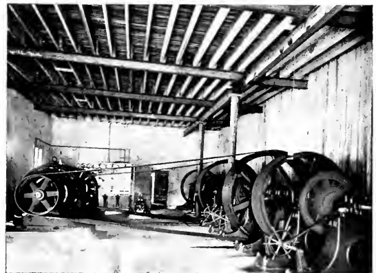
FIG. 3.—INTERIOR OF STATION.
